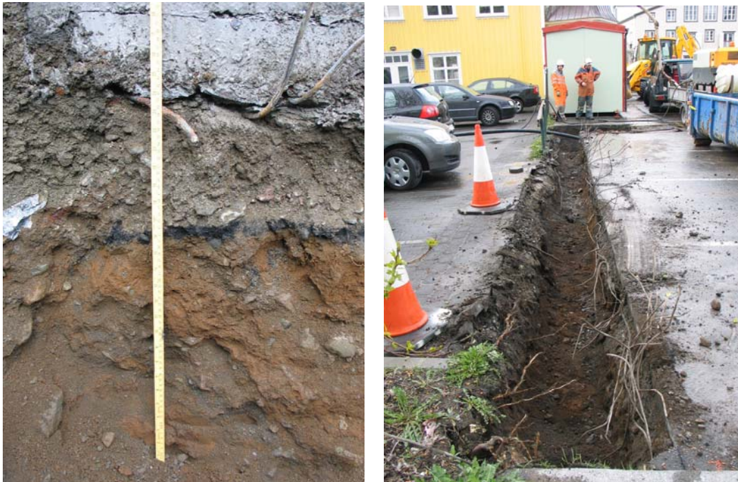
Figure 4. Section of trench [2i] – east facing (left); trench [2ii] looking south (right).
