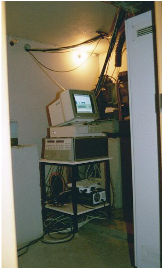
Figure 2.6 The data acquisition unit and computer in the control room.
