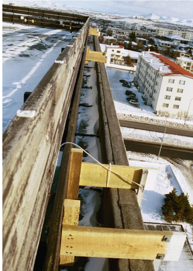
Figure 2.10 Location and fixture of tapping point plates on the southward side of the building.
