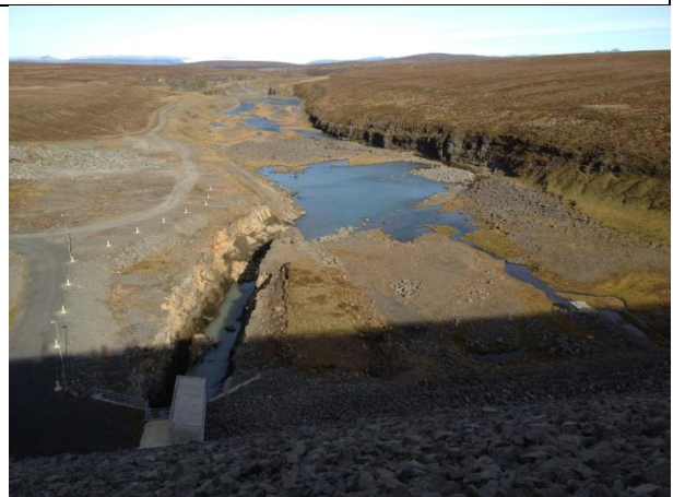
Photo 6: View downstream from Blanda dam with low level outlet; water is seepage and not an environmental flow release
