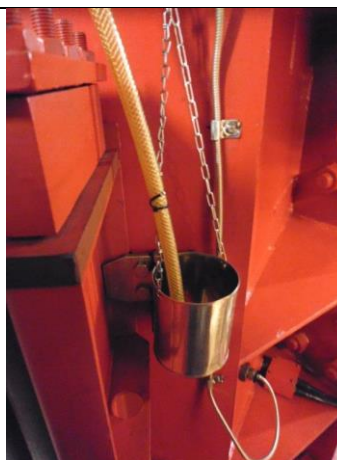
Photo 40: Oil drip catch in power station
