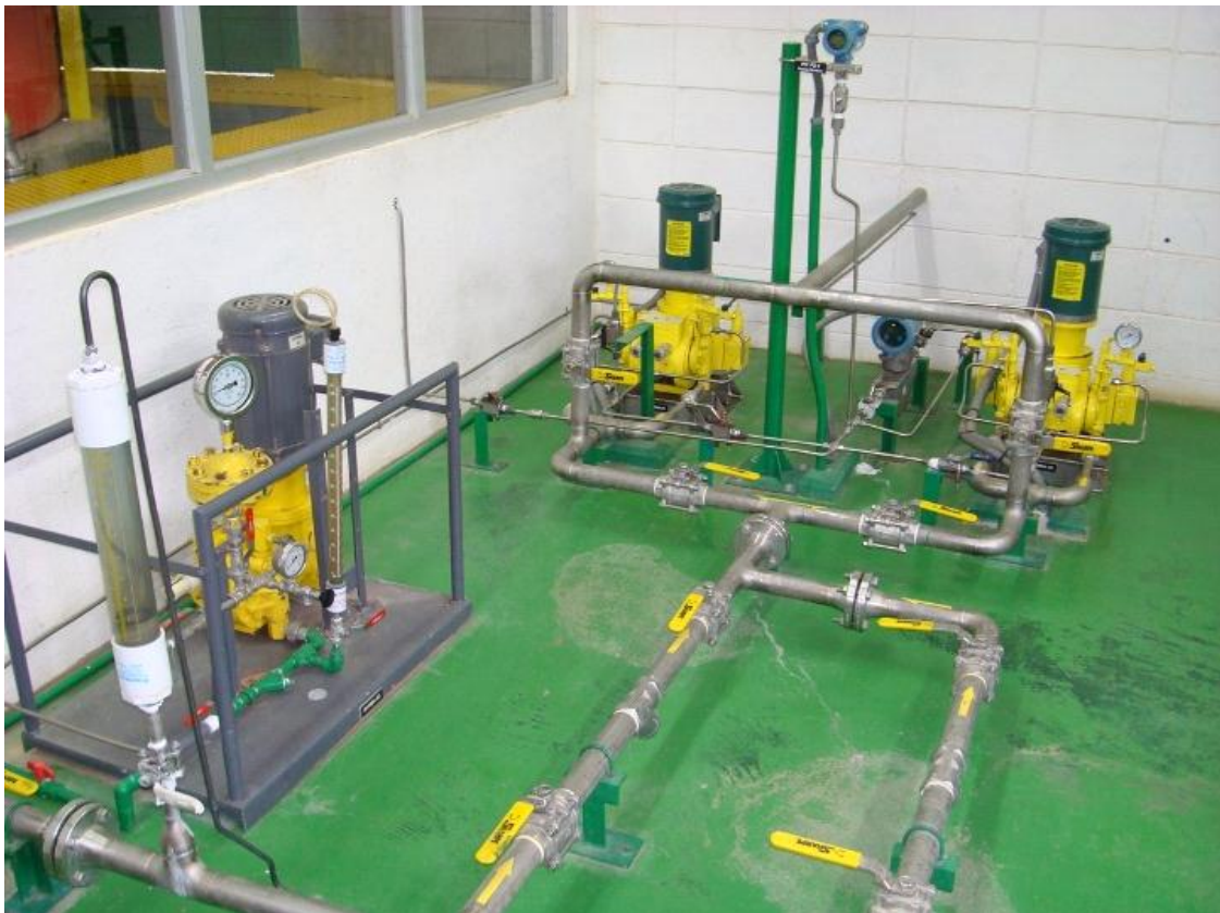
FIGURE 11: Metering Pumps at PGM-02. Photo by P. Moya
