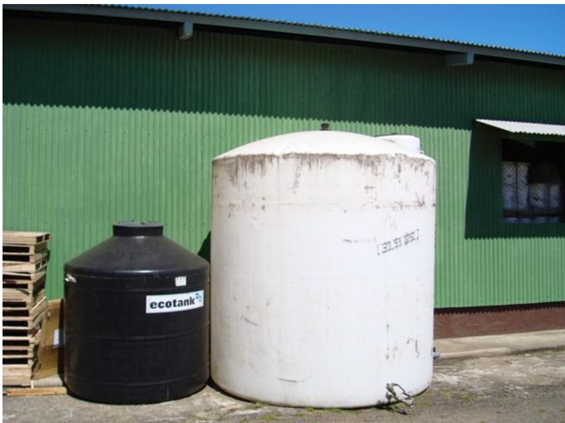
FIGURE 6: Inhibitor storage tanks. Photo by P. Moya
