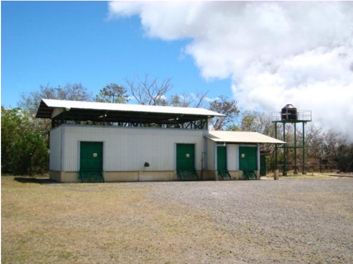
FIGURE 10: Neutralization System at well PGM-19. Photo by P. Moya
