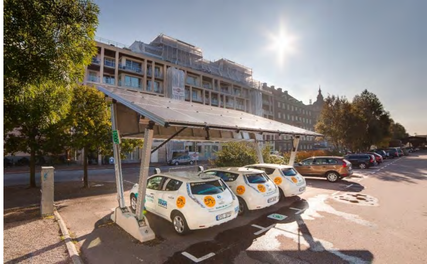
Picture 4: The solar carport in Helsingborg, Sweden; three EVs powered by 40m 2 of solar panels
