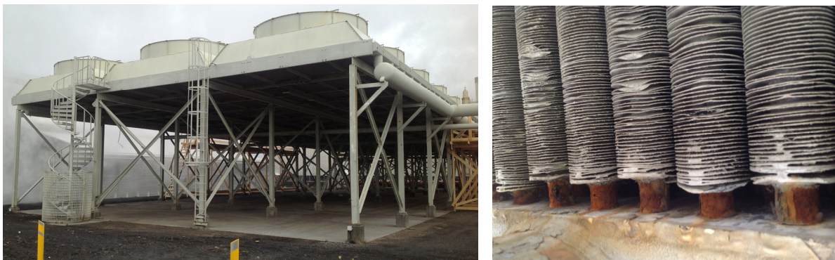
FIGURE 34: Air condenser and the leakage zone
