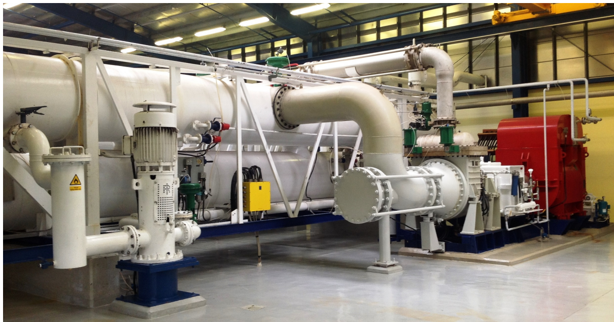
FIGURE 26: Binary Ormat unit at Svartsengi, water cooled condenser
