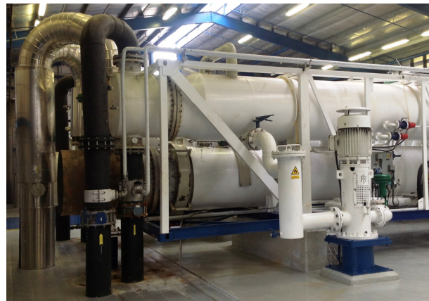
FIGURE 27: Isopentane pump belonging to the water cooled binary Ormat units at Svartsengi; it shows the Isopentane return pipeline from the condenser to the pump
