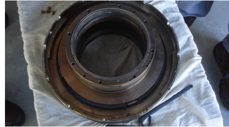
FIGURE 33: Mechanical seal, contaminated and damaged (Berlin binary cycle power plant)
