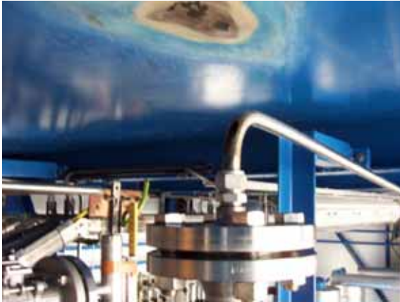
Figure 10 A pipe gave away in the hydrogen station from pressure and aggressive chemicals. Therefore a thorough and time consuming inspection took place in 2004 followed by and modifications of the design
