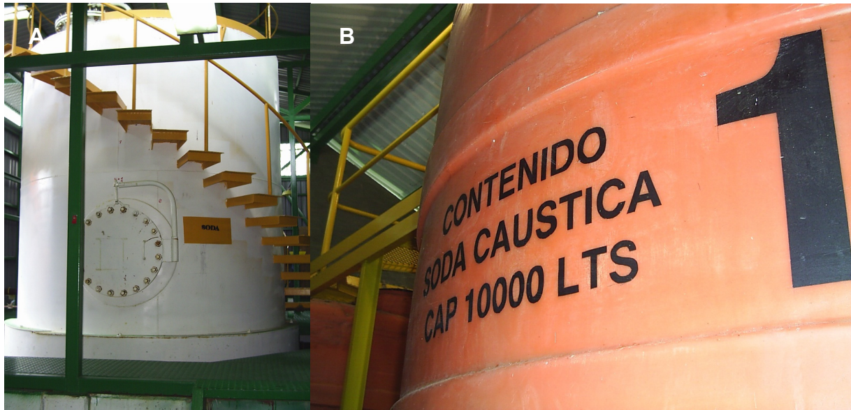
FIGURE 4: Storage tanks for neutralizing agent; a) Metallic tank of 25 m 3 ; b) Polyethylene tank of 10 m 3
