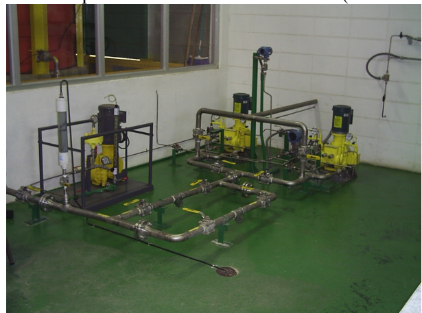
FIGURE 5: The low-pressure line, system pumps, high-pressure line and others accessories of the neutralization system
