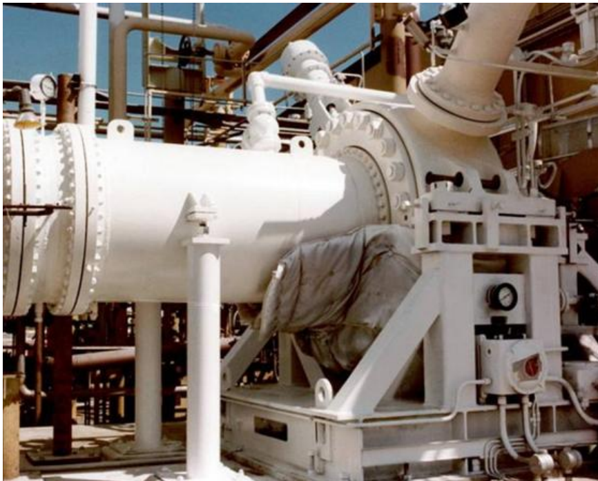
FIGURE 3: The Atlas Copco geothermal ORC turbine in East Mesa 1982
