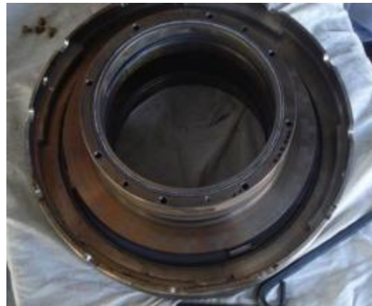
FIGURE 17: Mechanical seal contaminated and damaged (The Berlin binary power plant)
