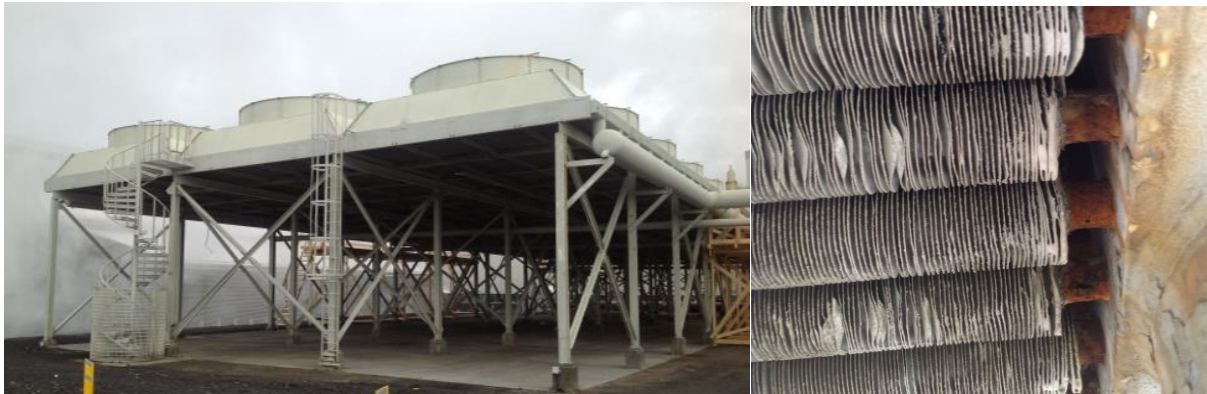
FIGURE 18: Air condensers and the leakage zone
