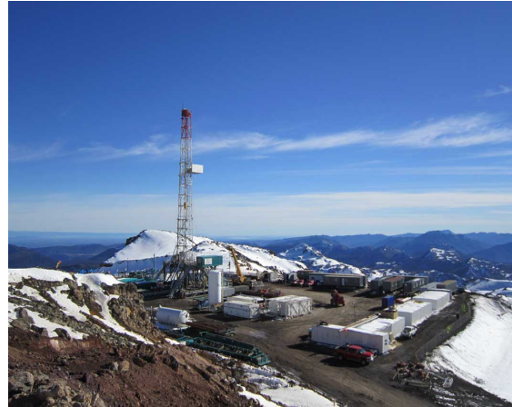
FIGURE 2: Geothermal project Cerro Pabellón. Source: Enel Green Power.
