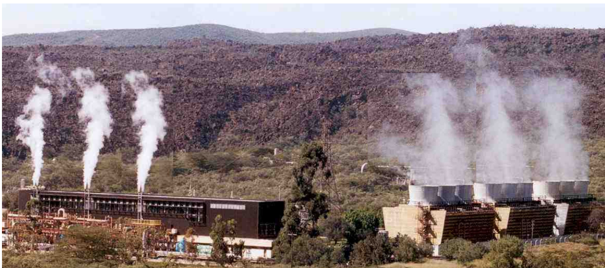
FIGURE 2: Olkaria I power station (45 MW)
