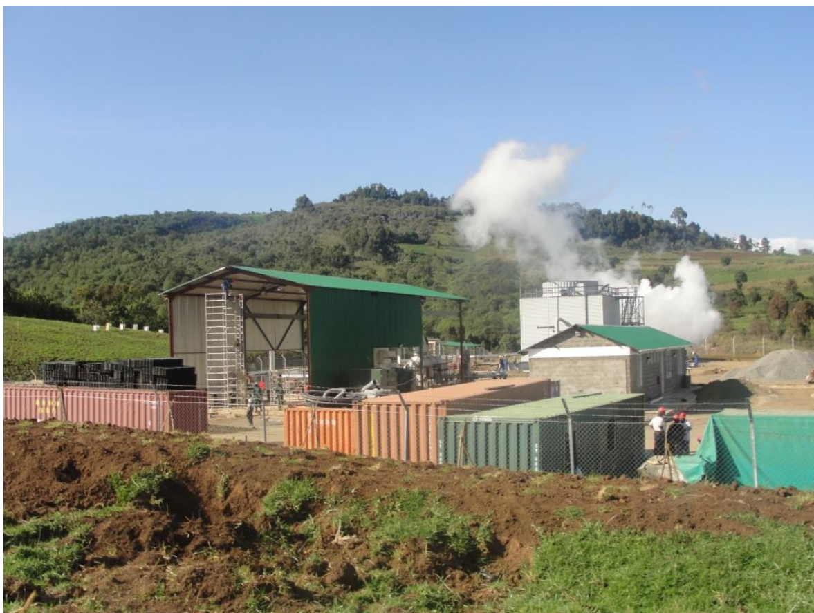
FIGURE 4: Eburru wellhead plant (2.5 MW)
