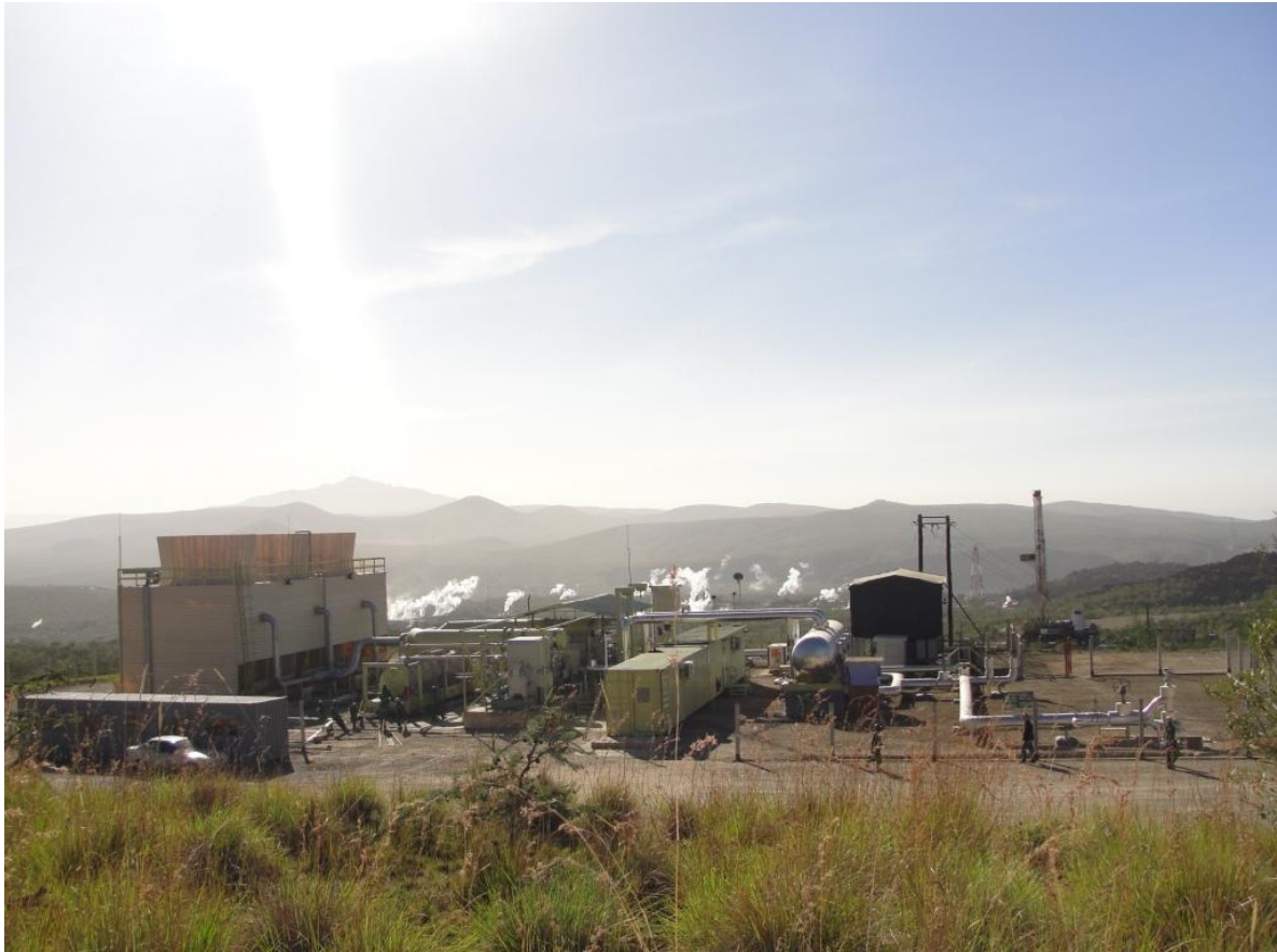
FIGURE 5: Olkaria wellhead plant (5 MW)
