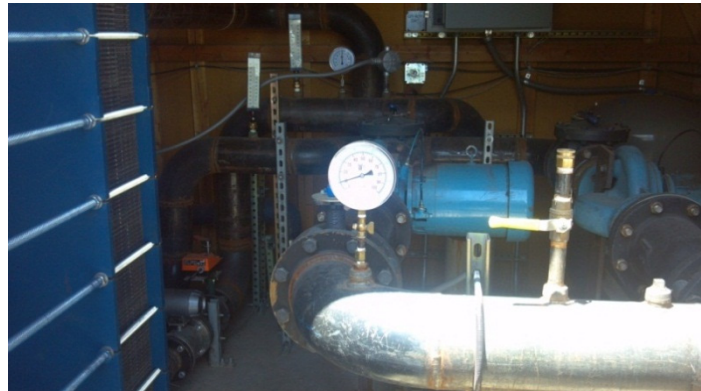
FIGURE 2: Klamath Falls heat exchange building. Some of the clients of the hot city water are 24 commercial and government buildings, greenhouses, sidewalk snow melt and a beer brewing company (Chiasson, 2006)
