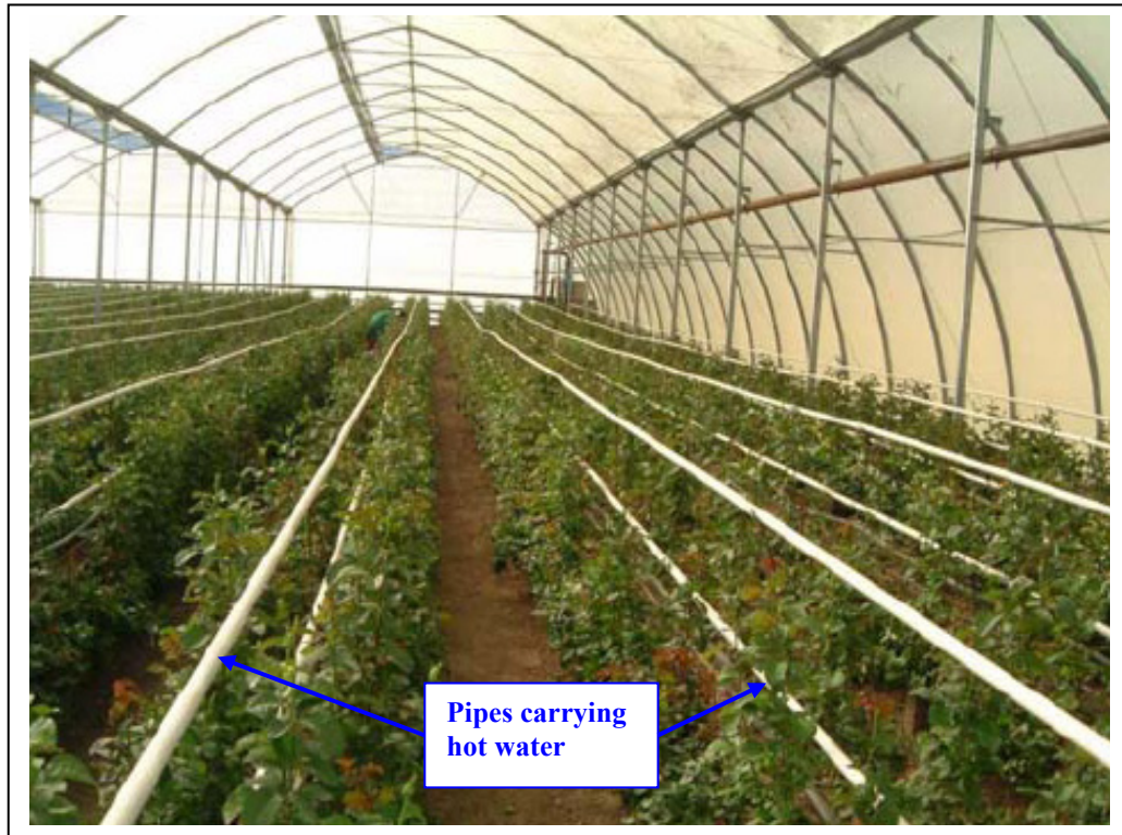
FIGURE 6: Geothermal greenhouse heating at Oserian Company, Kenya.
