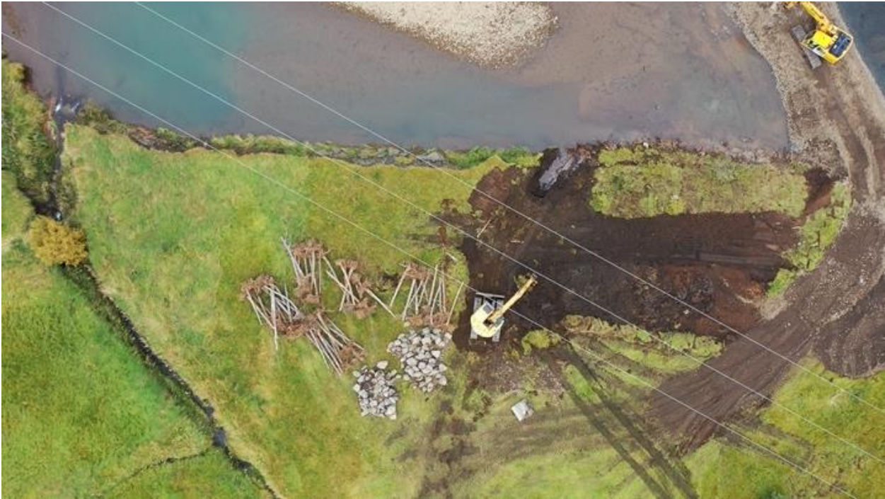
Figure 22. Aerial photo over the area where the material used for the riverbank restoration is used e.g. big logs and stones (McGowan Environmental Engineering Ltd).
