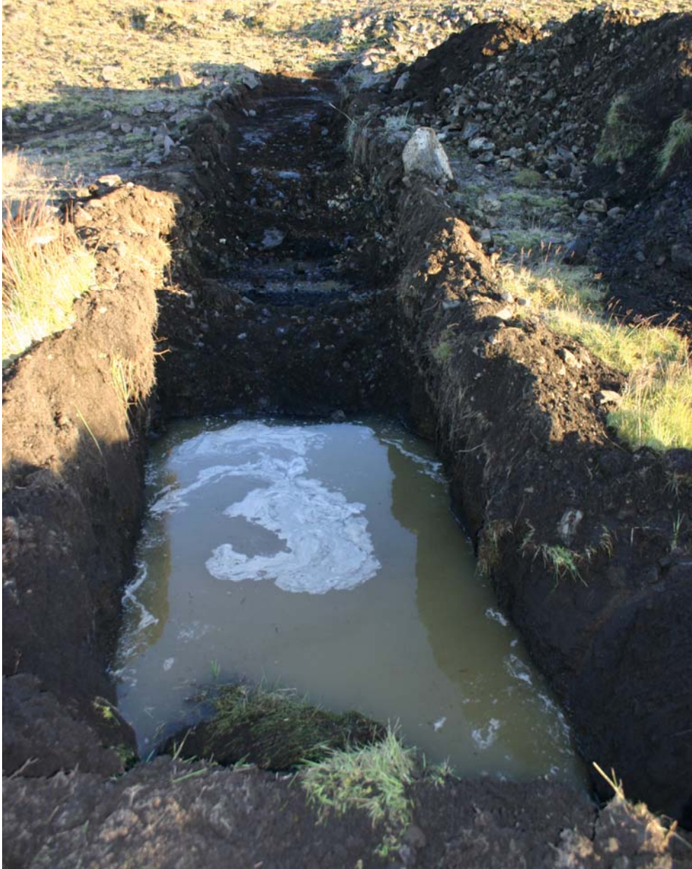
Figure 2-5. Fissure trench AK 3 in process of excavation. The inflow of groundwater made the study difficult
