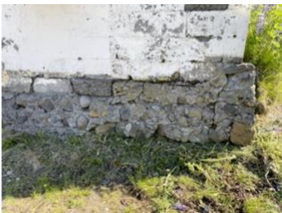
Fig 1. The typical foundation beneath an old building built around 1900. The rocks can be seen from the outside and the concrete grouting in between, often called a mortar wall.
