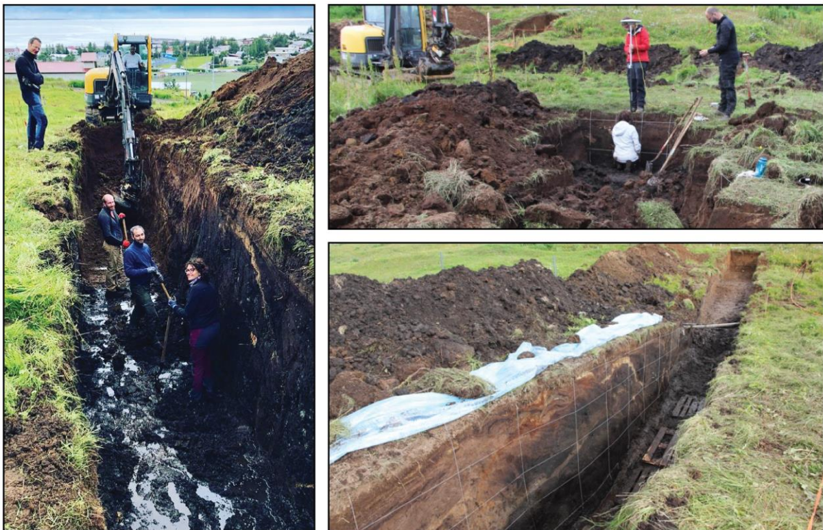
Figure 2: Field pictures of the excavation of trench Tr1 in Traðargerði. Left. SW looking view of Tr1. Bottom right. NW looking view of Tr1. Top right NW looking view of secondary trenches just east of the main trench Tr1.
