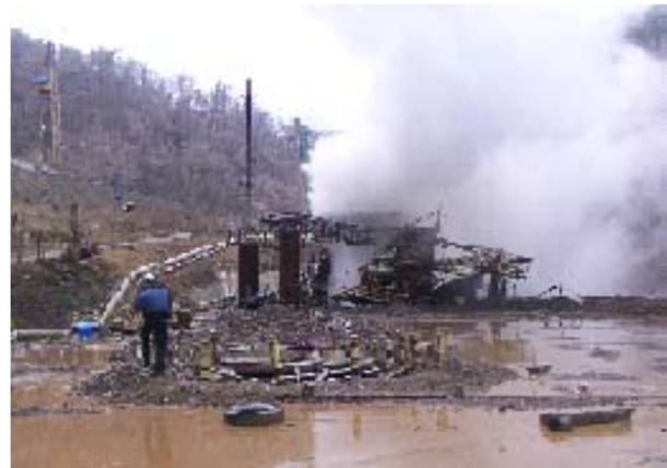
FIGURE 14: View of well 5R-12D that blew out and toppled the rig (Jumawan et al, 2005)
