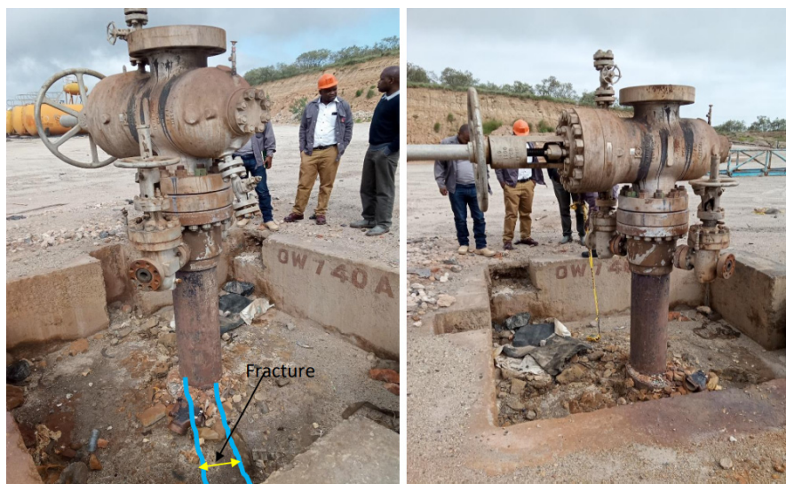
FIGURE 2: Situation at well OW-740 at the initial stages of steam leakage development (July 2019)
