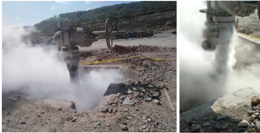
FIGURE 3: Steam leakage at later stages of development
