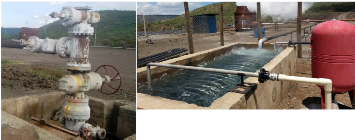
FIGURE 8: Low enthalpy well as the heat source and a simple helical coil heat exchanger
