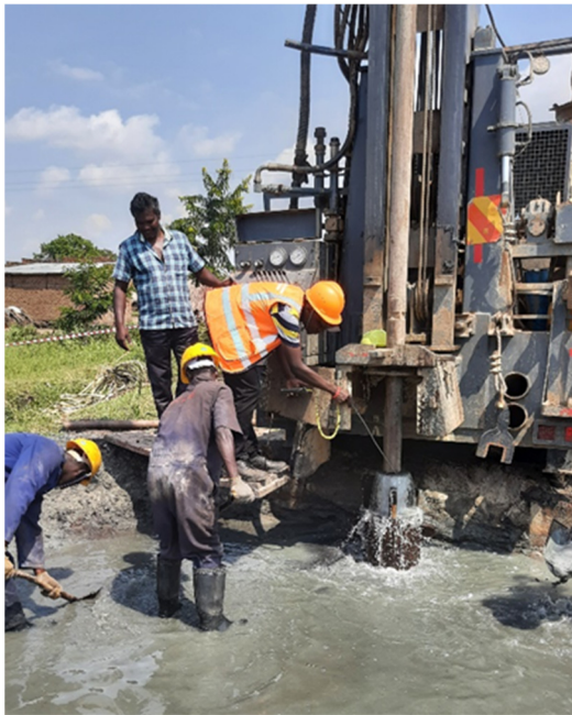
FIGURE 9: TGH drilling at Panyimur intercepting of fluid of at a temperature in PAN-7
