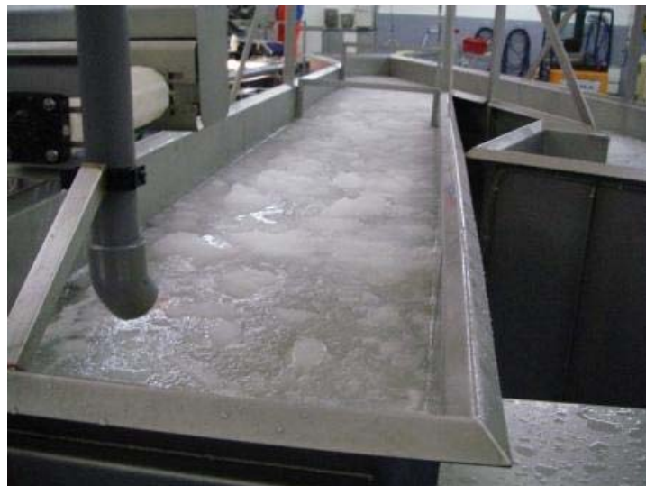
Figure 12. Slurry ice cooling tank, the inlet is visible to the left.
