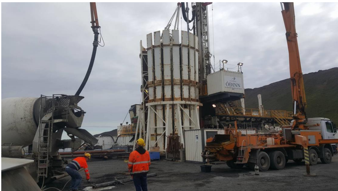
Figure 1. The cement truck and crew at work the morning of August 10 th .
