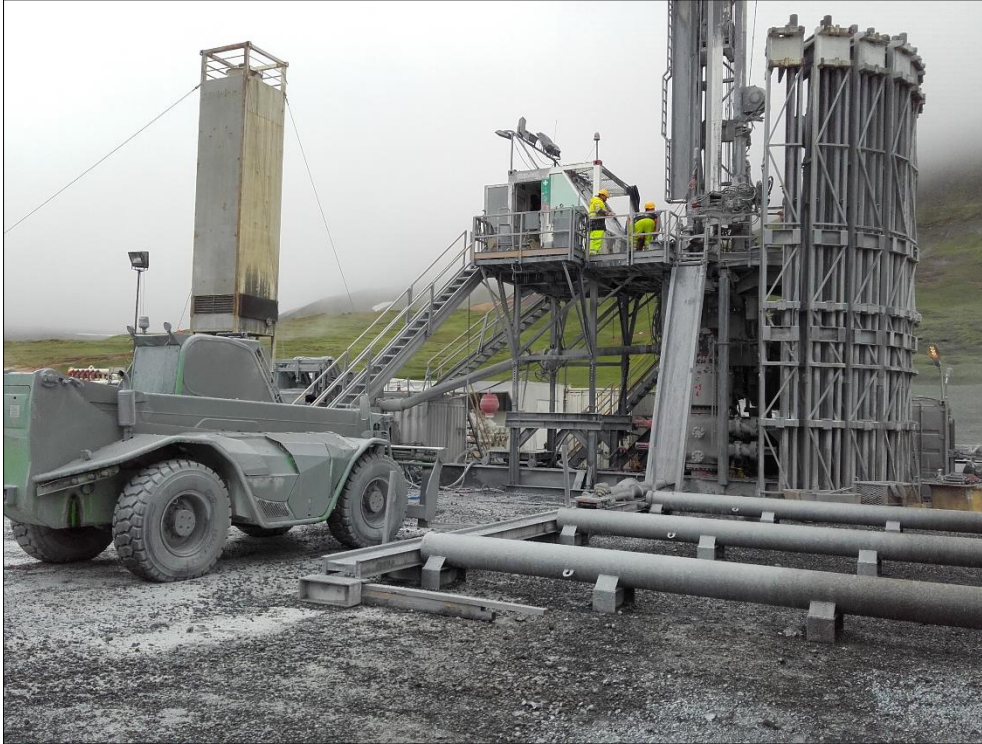
Figure 1. Mud and debris at well pad A after a blow-out from PG-10 at 5:30 am this morning.
