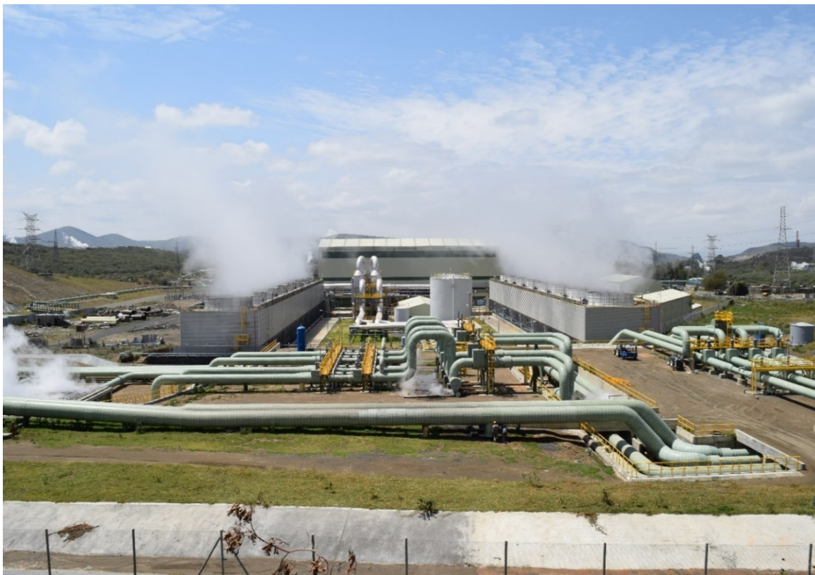
FIGURE 5: A view of Olkaria IV power plant located in Domes area
