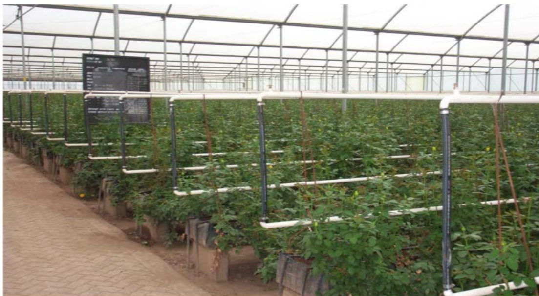
FIGURE 9: Oserian greenhouse heating using hot geothermal fluids
