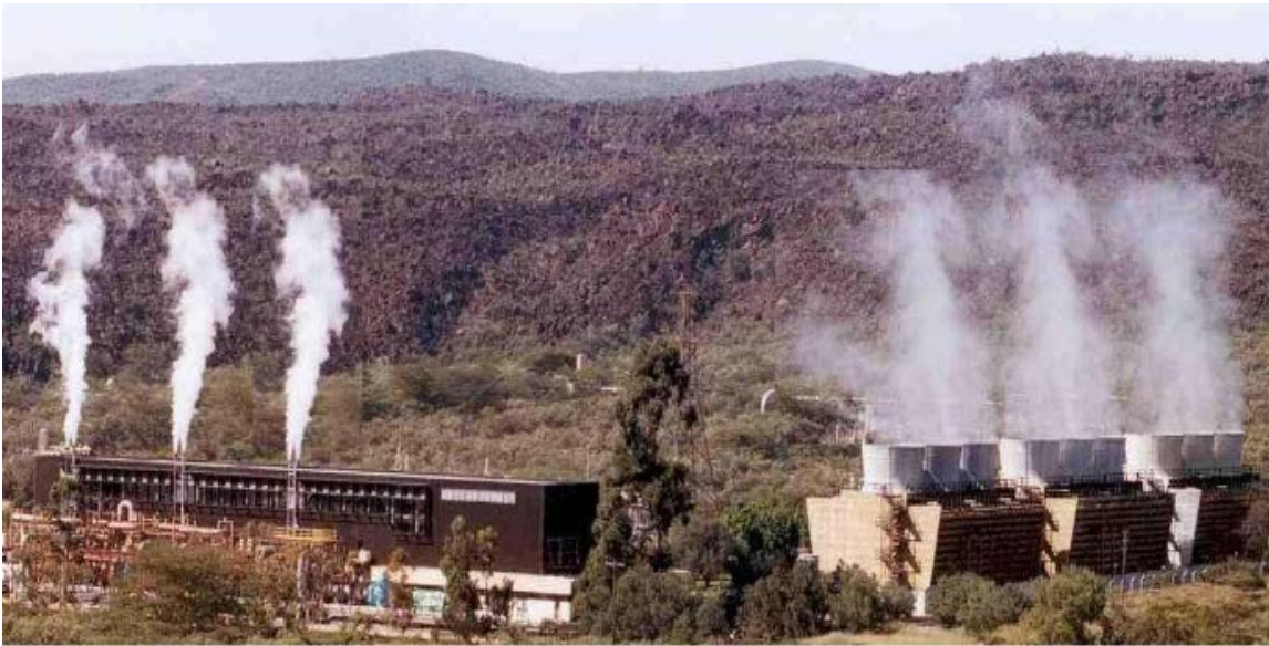
FIGURE 3: A view of Olkaria I Power plant located in the Olkaria East Production Field
