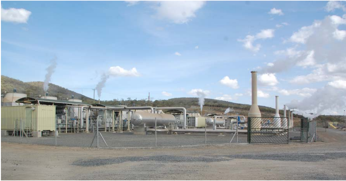
FIGURE 7: OW-914 wellhead generating units with an aggregate capacity of 29.3 MWe
