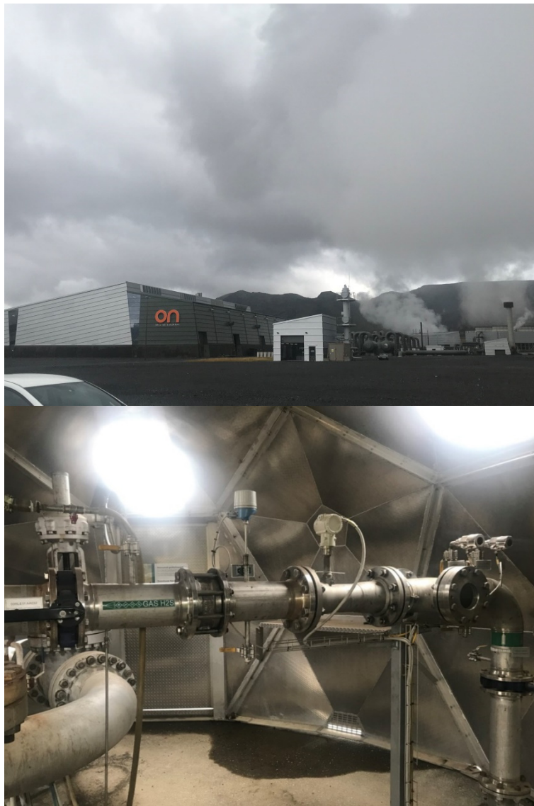
FIGURE 39: The CarbFix project at the Hellisheidi geothermal power plant, Iceland
