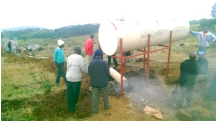
FIGURE 7: Water condensing units at Eburru
