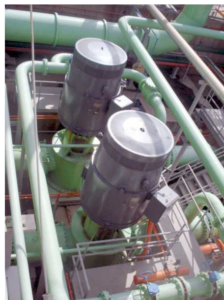
FIGURE 6: Circulation pumps in the Berlin power plant, unit 1
