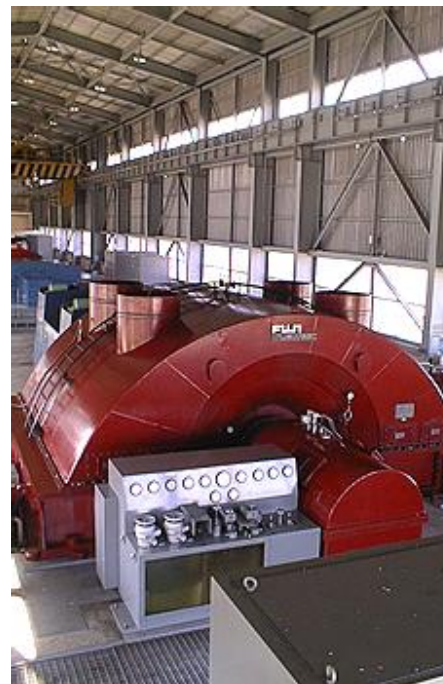
FIGURE 4: The generator of unit 1, Ahuachapán
