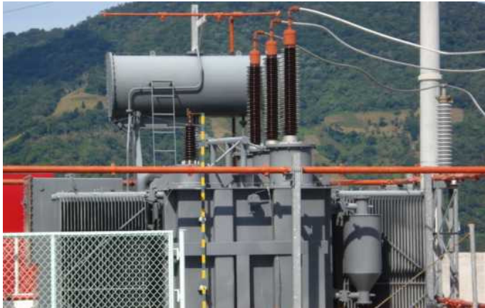
FIGURE 5: Unit transformer, Berlin unit 3
