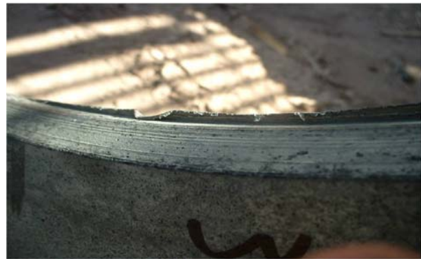
FIGURE 33: Erosion in the inner edge of an orifice disc used to measure steam flow at Cerro Prieto geothermal field, Mexico (Canchola and Sánchez, n.d.)
