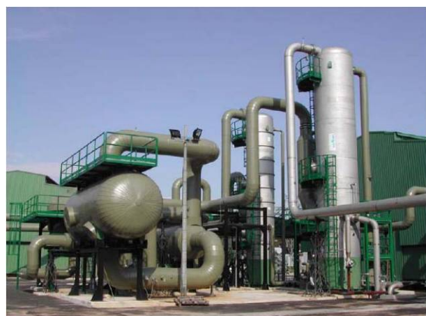
FIGURE 25: A picture of the AMIS H_2S abatement system installed at the Travale 4 geothermal power station (IEA, 2006)
