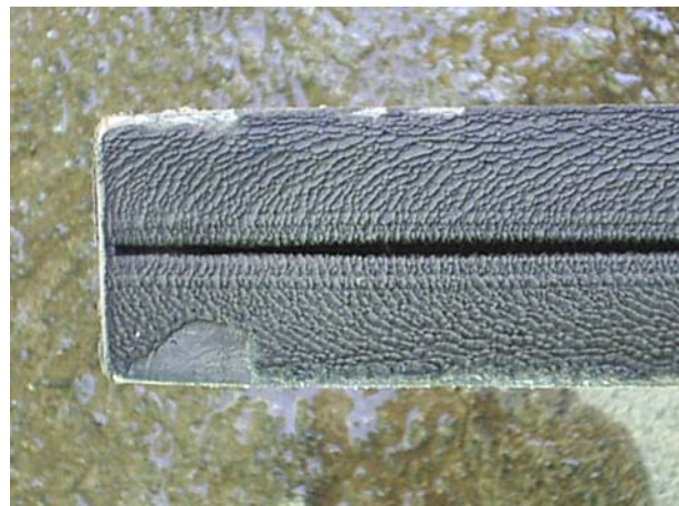
FIGURE 30: Deposition in the upstream face of an annubar flowmeter in a reinjection line, Ahuachapán
