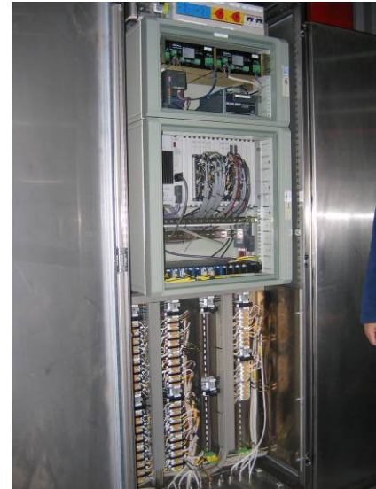
FIGURE 19: Outdoor pressurized electronic panel with inner cabinet to protect a remote I/O rack at the Nesjavellir power plant, Iceland
