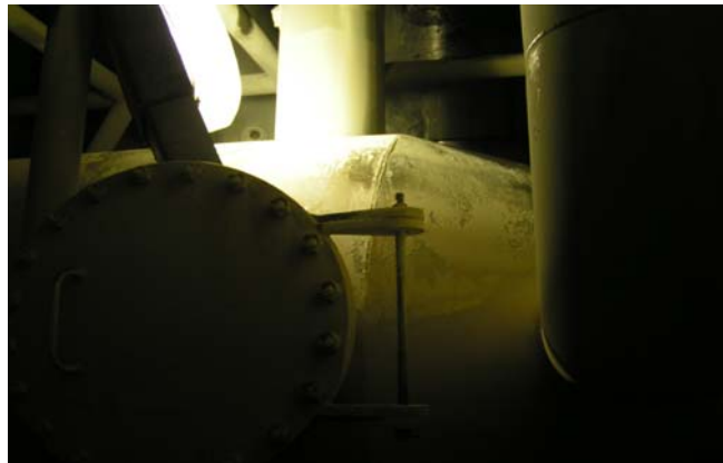
FIGURE 11: Deposits in main condenser
