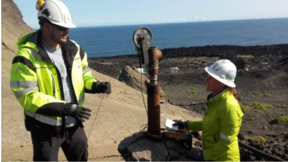
Figure 7. Picture showing Tobias B. Weisenberger and Erica Massey installing a temperature and pressure monitor string in SE-1 on August 19 th , 2017 (image source: AB).
