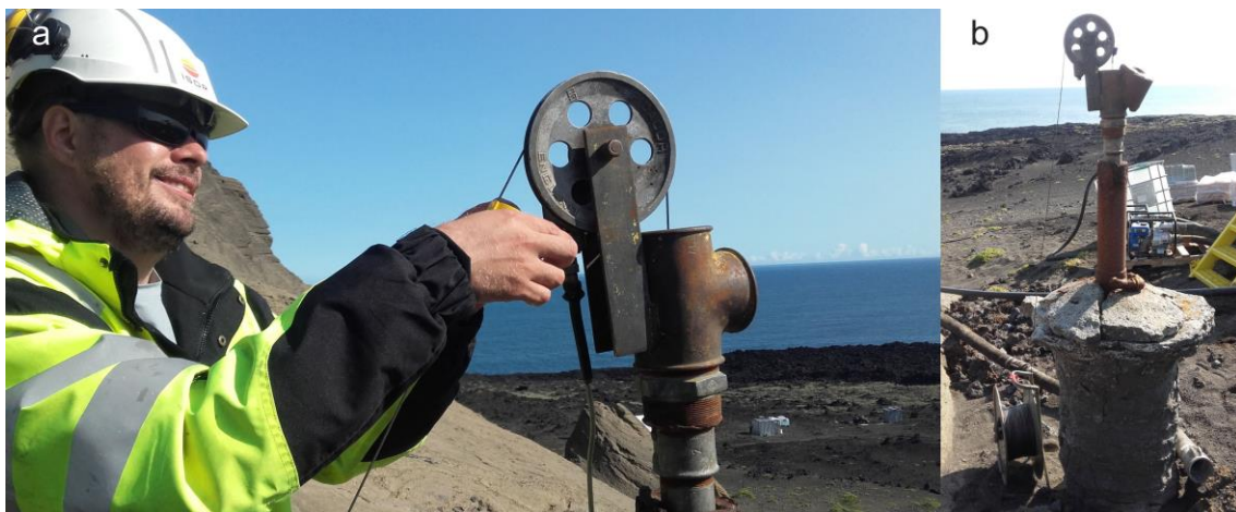
Figure 33. Photograph showing installation of the pressure and temperature monitoring string in SE-01 (Table 12) (photos: AB).
