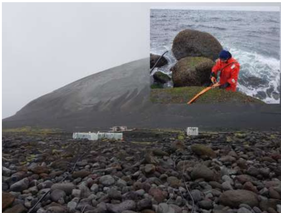
Figure 2. The supply of water was the greatest challenge in the early part of the project. This problem was finally brought under control by having two designated water men operating an array of pumps. The inset shows Einar Sindri on beach fastening pumps to large boulders. (photos Sveinbjörn Steinþórsson).
