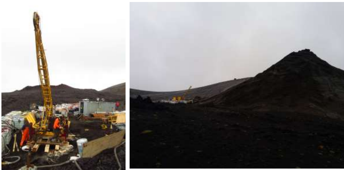
Figure 2. Picture showing the rig orientated along the drilling direction (left picture) and the angled mast (right picture) (image TBW).
