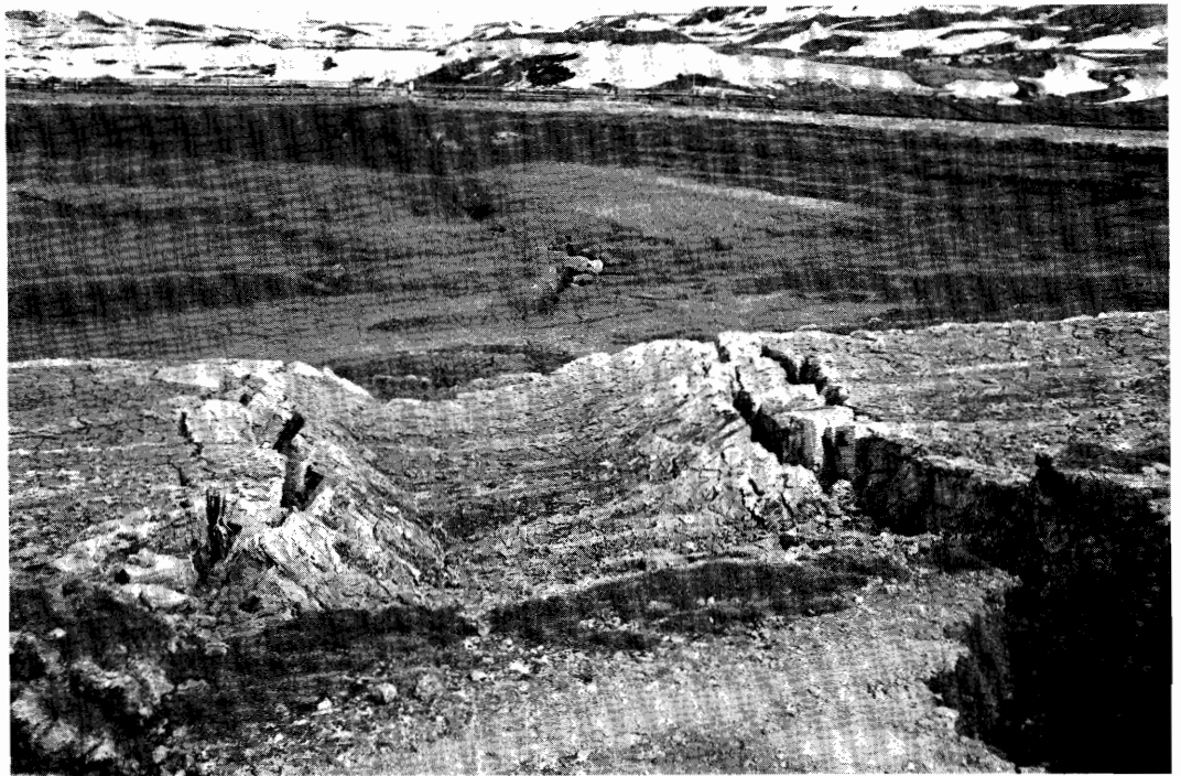
Fig. 7: One of the empty diatomite reservoirs at Bjarnarflag. This one was emptied through the fissure seen on the bottom of the reservoir.
