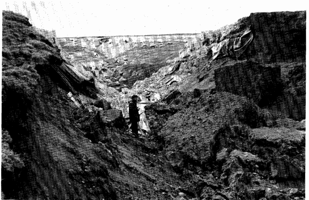
Fig. 8: Another diatomite reservoir was emptied through this breach in the earth dam caused by a fissure that can be seen in the background running through the reservoir bottom. The polythene sheet can be seen on both sides of the breach.
