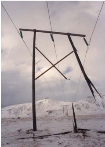
Fig. 8: Tower in a 132 kV line, hit by lightning.
