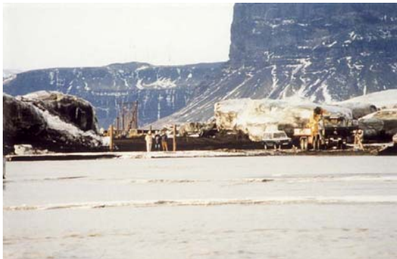
Fig. 6: Consequence of “jökulhlaup”. Reconstruction of the line (132kV) has started between huge icebergs left by the flood.
