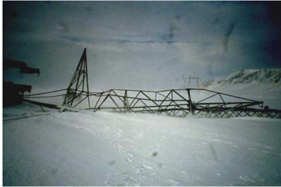
Fig. 10: Collapsed tower in a 220 kV line.
