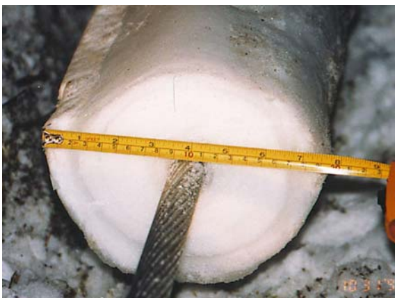
Fig. 11: Wet snow icing on a conductor.
