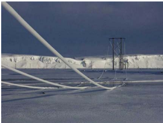
Fig. 15: Wet snow iceload on a river crossing span.
