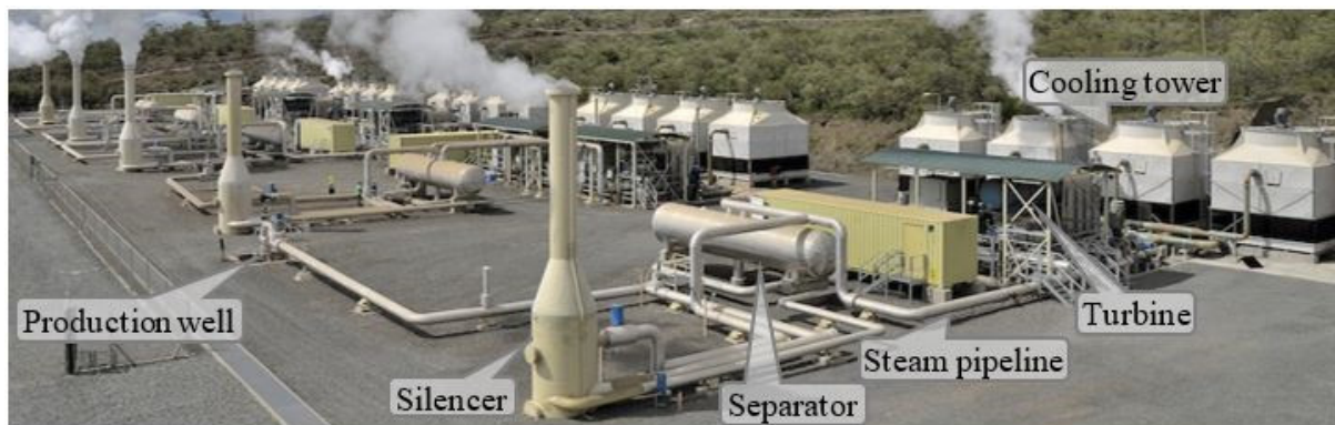
FIGURE 1: OW 914 Wellhead power plant
