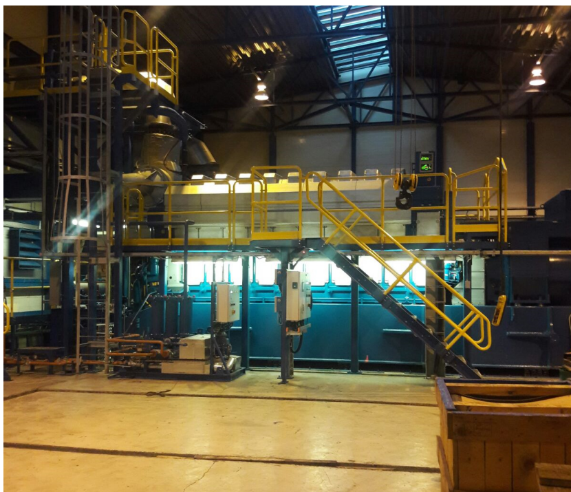
FIGURE 2: The 3.85 MWe Wartsila Engine installed in 2017
