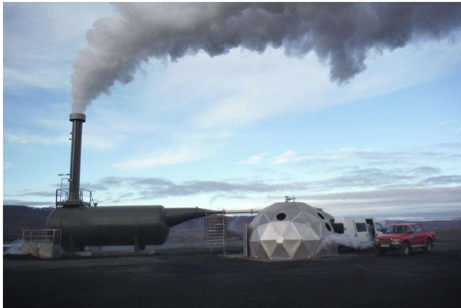
Figure 10: A geothermal well with silencer, during testing.
