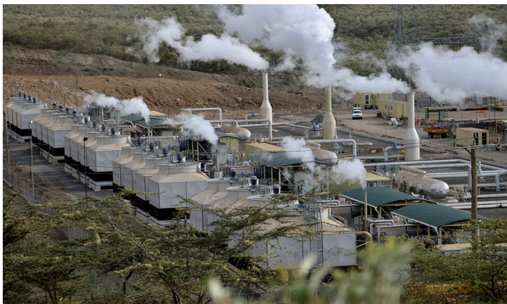
FIGURE 3: 27.8 MW WHP located at OW 914 well pad in Olkaria, Kenya (courtesy of Lýður Skúlason, 2017)
