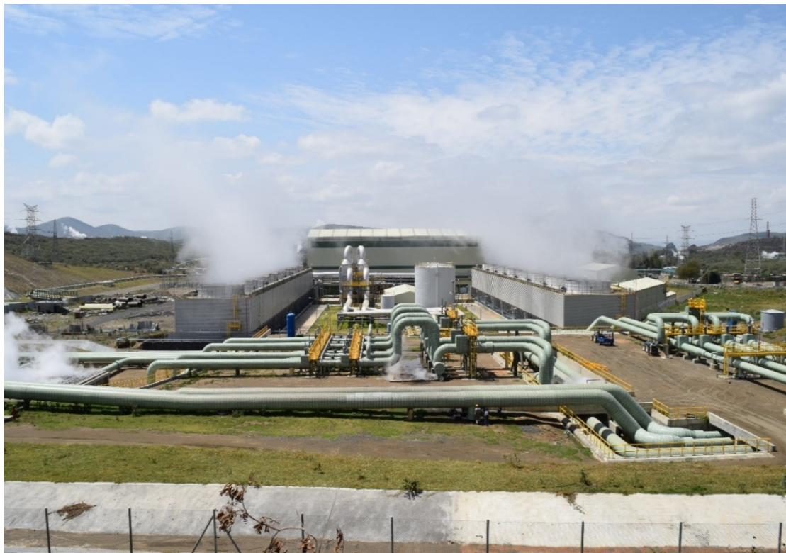
FIGURE 5: Olkaria IV power plant located in Domes area
