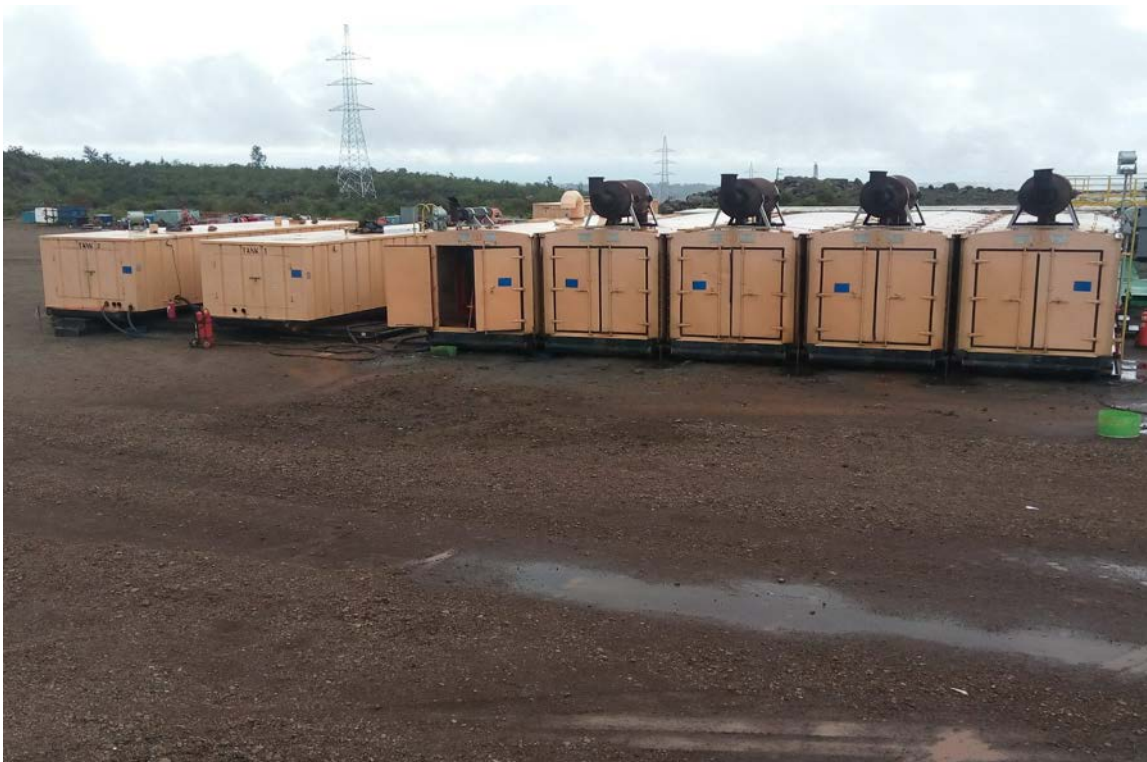
FIGURE 1: Diesel tanks and power generating unit
