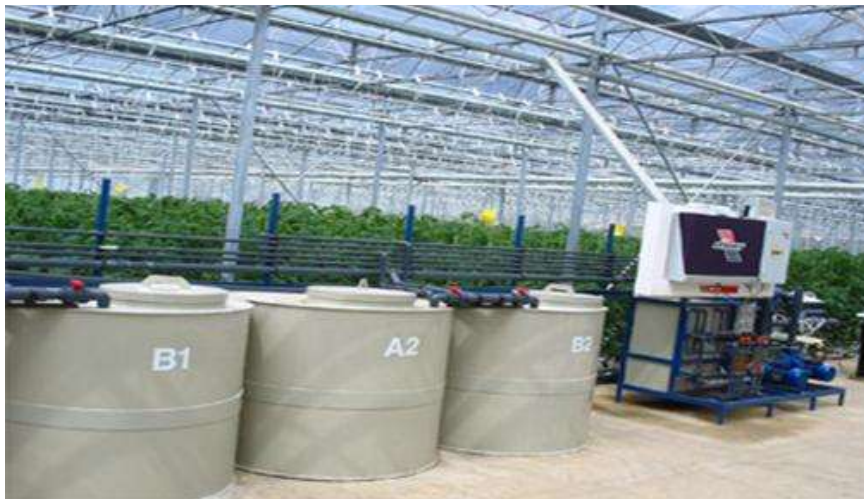
Greenhouse heating – Livada, Bihor County
