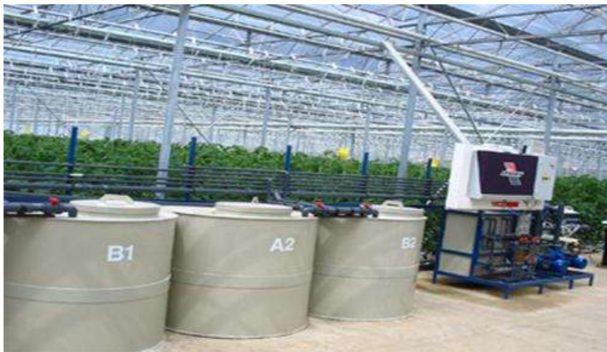
Greenhouse heating – Livada, Bihor County
