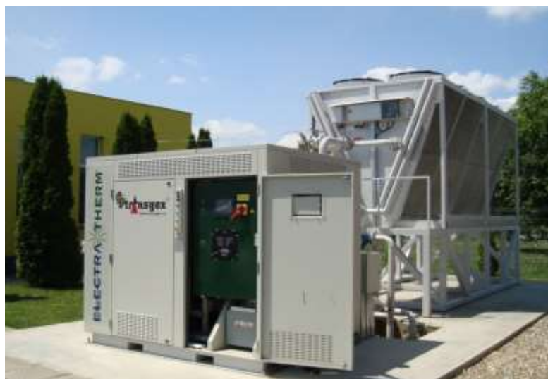
50 kW Binary Cycle ORC Geothermal Power Plant installed in Oradea by Transgex Company
