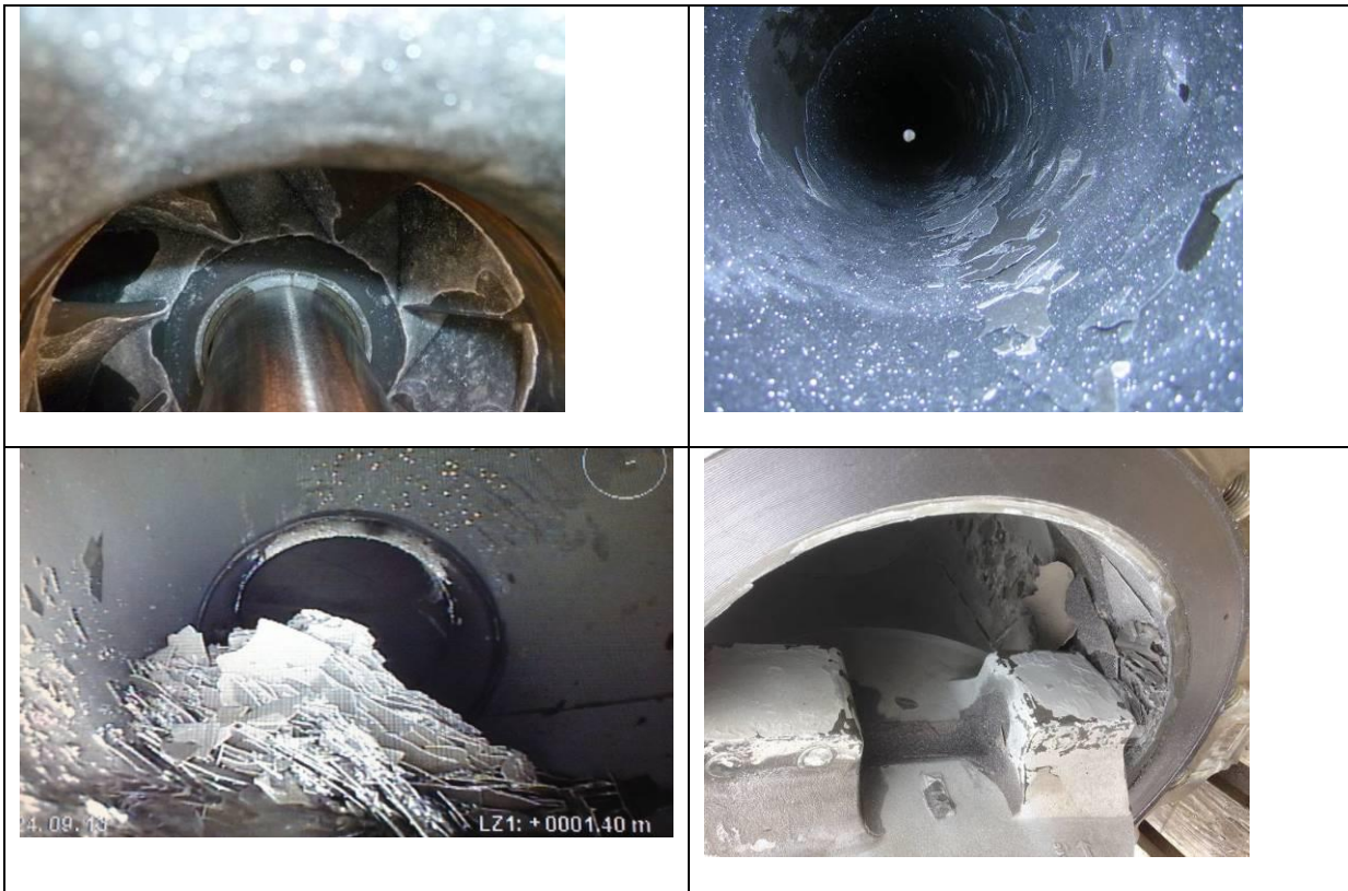
Figure 23 Carbonate scalings in (a) a pumping stage of the ESP (b) rising pipe, (c) surface pipe and (d) heat exchanger of four geothermal power plants located in the Bavarian Molasse Basin.
