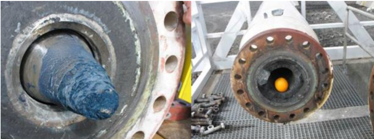
Figure 12 Sulphides scales precipitated in one year. To the left the scales (mainly ZnS covered by Cu-sulphide) coats the fluid-flow control valve (14 cm long). To the right the scales (mainly ZnS) coats the inner surface of the pipe (7 cm thick).
