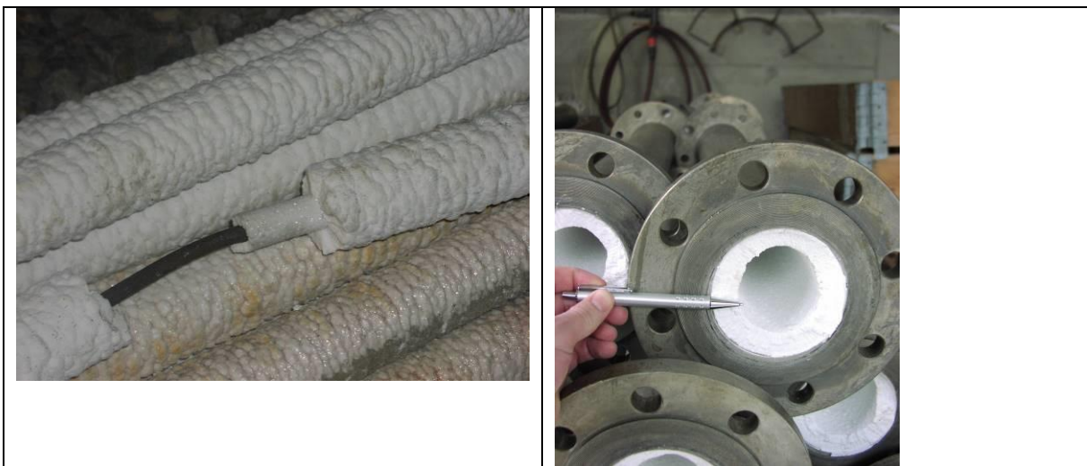
Figure 22 Carbonate scalings in production wells of geothermal plants in the Pannonian basin; left: massive calcite precipitations caused by the ascent of thermal waters during a defect in the inhibitor injection hose; right: massive calcite precipitations formed by the ascent and degassing of thermal water, which are removed by periodic acidification
