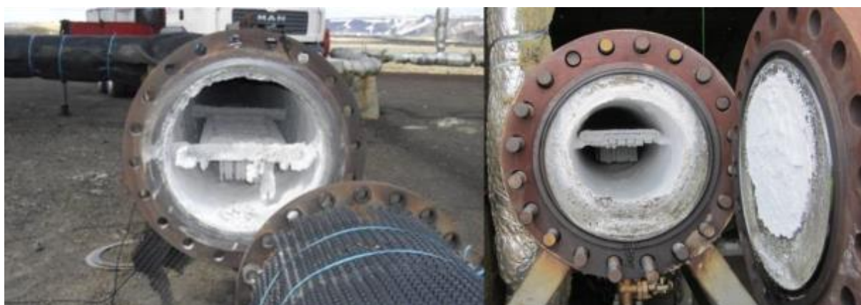
Figure 11 Silica scaling occurring inside geothermal pipes after 14 days of use. Samples for corrosion testing can be seen totally sealed by the scale.
