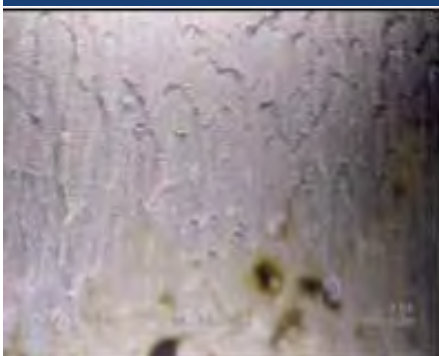
Barite scales on injection pipe (80 m b.s.) (Scheiber et al., 2014)
