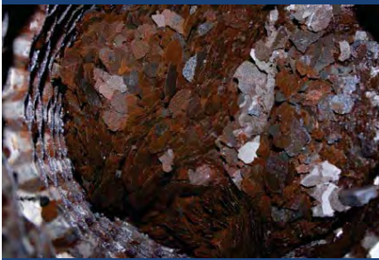
Barite and Celestite scaling in heat exchanger (Degering et al., 2008)
