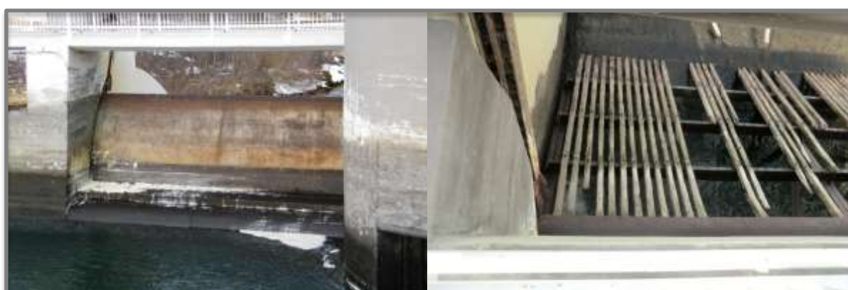
Figure 29: The flood-sluice-gate with damaged downstream apron made of wood-staves
