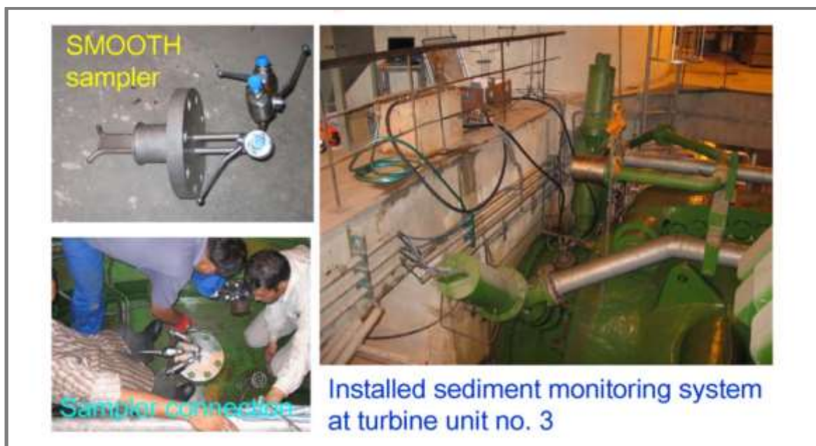
Figure 32: Installation of a SMOOTH sediment monitoring rig at a high head Francis turbine in India
