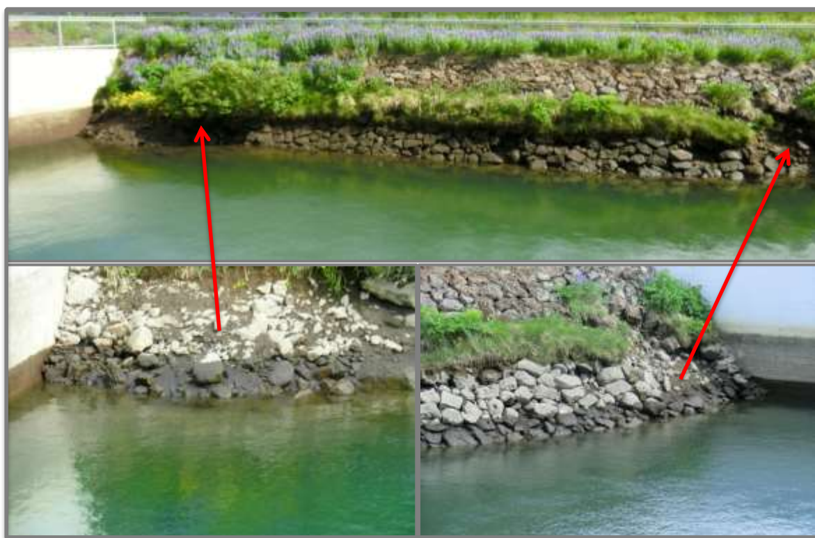
Figure 26: Damages of the stone masonry lining along the right bank of the forebay
