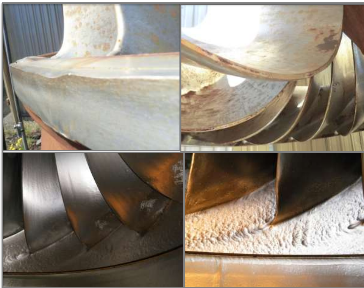
Figure 17: Upper: replaced runner from Laxá 2 with signs of sediment-induced wear. Lower: the runner of Laxá 3 from an inspection of the turbine on 5 th April 2011 (Ref. 3).
