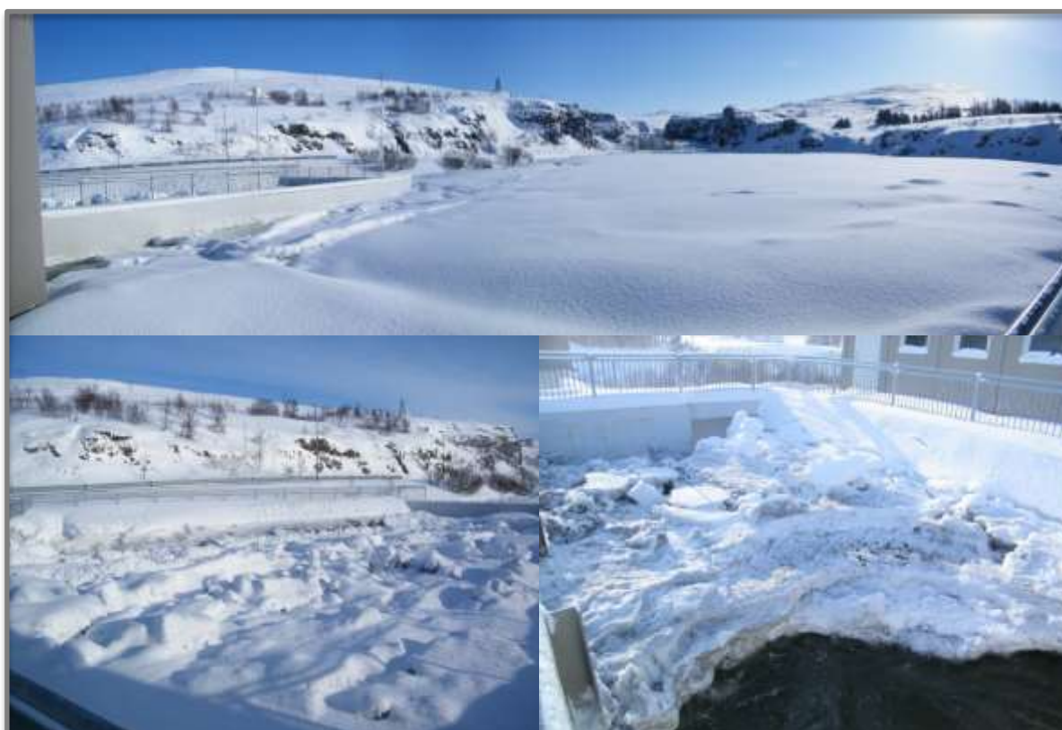
Figure 28: Ice action in the head-pond and the forebay of Laxá II dam (Ref. 3)
