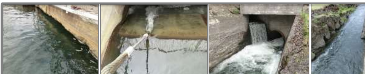
Figure 9: Overflow gate for passage of ice at the old intake location to Laxá 1 HEP
