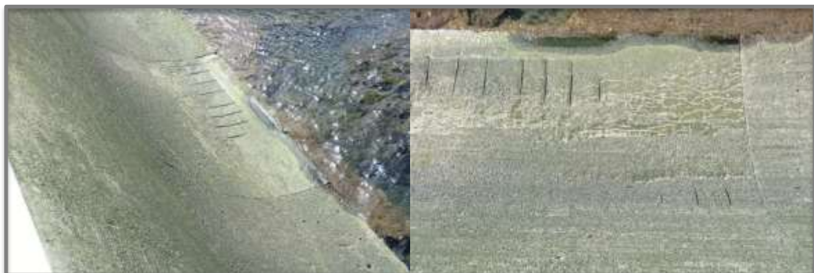
Figure 16: Damages at the flip bucket of spillway at Laxá II dam
