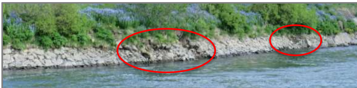
Figure 27: Damages of the stone masonry lining along the right bank of the head-pond
