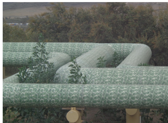
FIGURE 12: Camouflaged green and beige steam pipes
